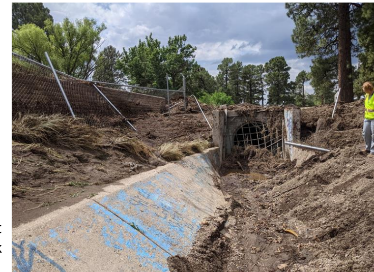
Damaged Fanning Wash channel at Bushmaster Park
